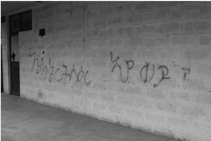
Figure 4.2. Slogan written on wall of Gerhu Sirnay Hospital, which was destroyed by the Eritrean Defence Forces
